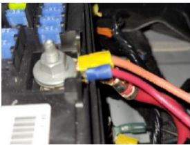
Bolt on top of fuse box provides 12v, and nut holding fuse box down in back provides ground
