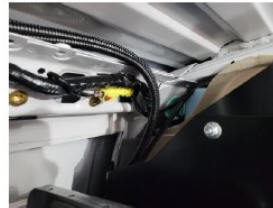
VTM harness routed up street side B pillar
