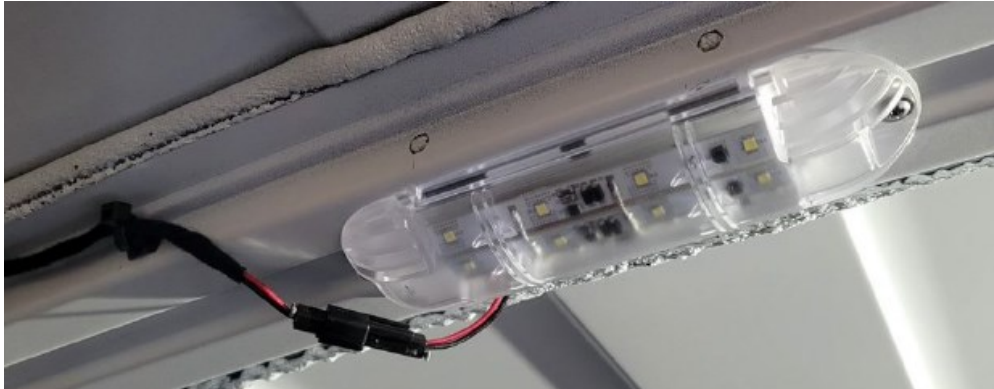
Module LED Light Installed
