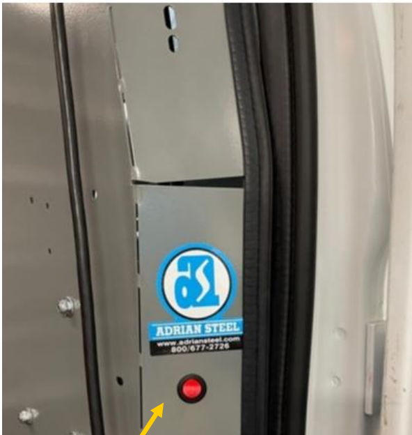
Steel partition hole behind passenger seat
