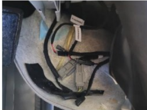
VTM connection point
