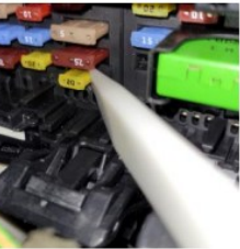
20amp fuse does not fit anything in vehicle, use a spare 20amp fuse from BCM
