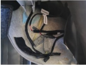
VTM connection point
